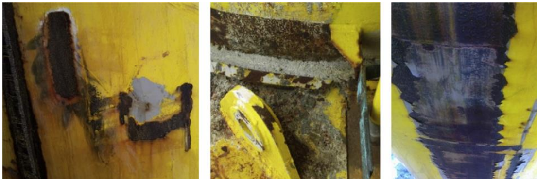
Figure.2. Significant metal losses caused by corrosion on offshore platforms[5].
